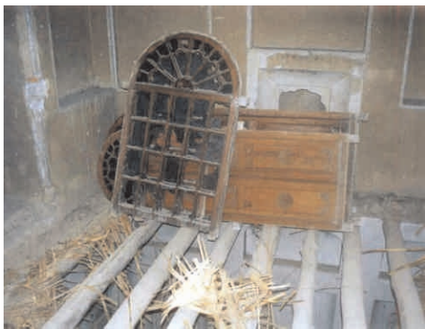
Destruction of cultural heritage...interior of the House of Mirza Abbas Nuri (Mirza Buzurg) during demolition, Tehran, June 2004.
