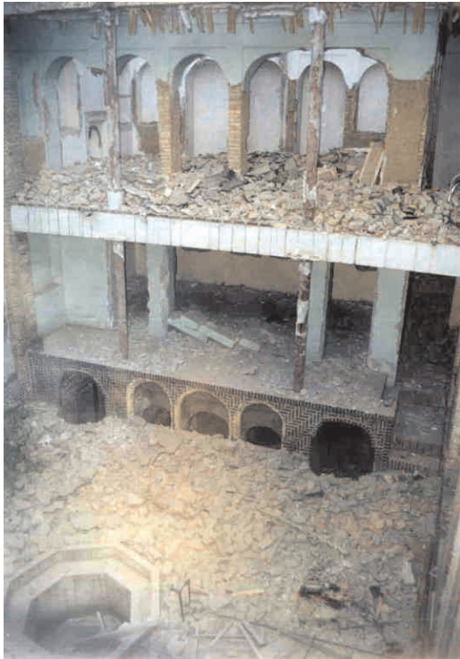
Demolition underway...the House of Mirza Abbas Nuri (also known as Mirza Buzurg), Tehran, Iran, June 2004.
